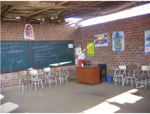
A leaky classroom
